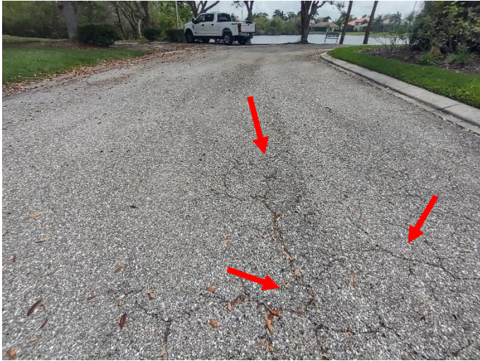
Typical Alligator Cracking & Raveling – Grande Vista Court
