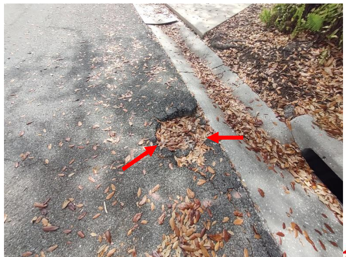
Typical Asphalt Depression – Pennyroyal Rd
