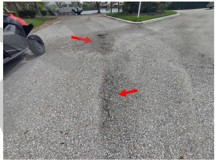
Typical Asphalt Raveling – Grand Vista Ct
