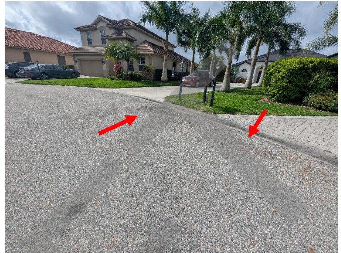
Typical Asphalt Raveling – Bay Ridge Way
