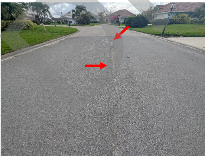
Typical Asphalt Raveling – Palmetto Point Ct
