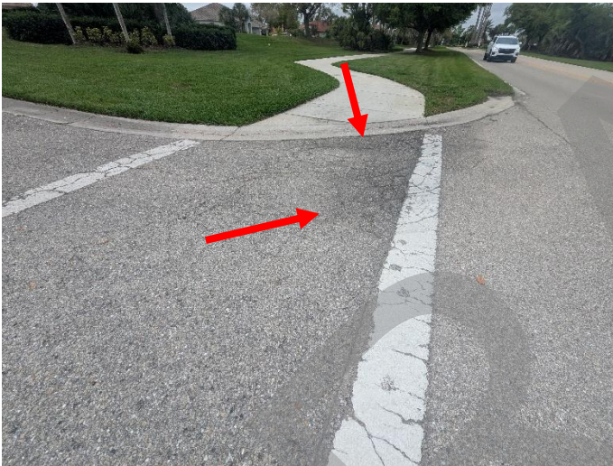
Typical Alligator Cracking – Lakes Ct
