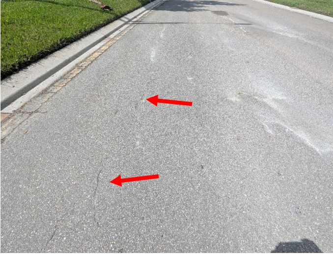
Typical Longitudinal Cracking – Riverwood Dr
