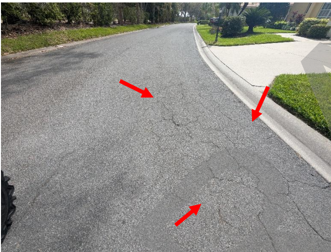
Typical Alligator Cracking - Bay Ridge Way
