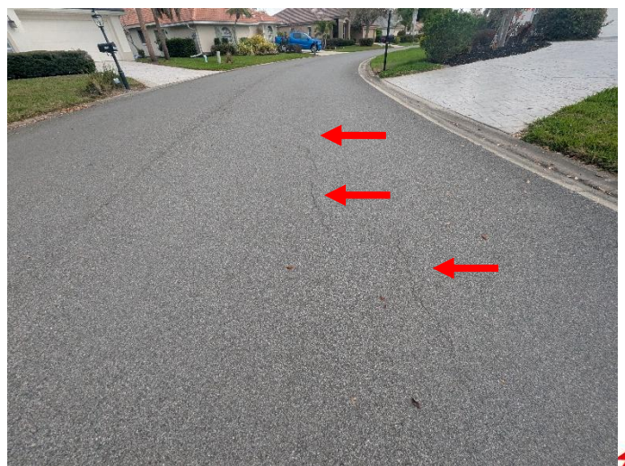
Typical Longitudinal Cracking – Long Lake Ln
