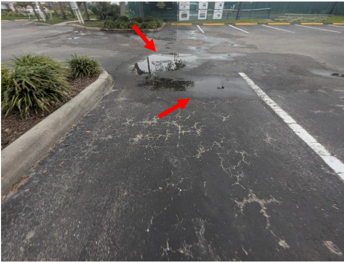
Typical Asphalt Depression – SW Parking Lot
