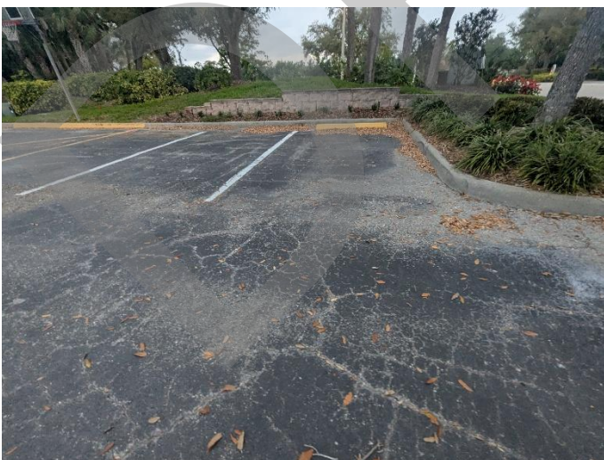
Typical Alligator Cracking – SW Parking lot
