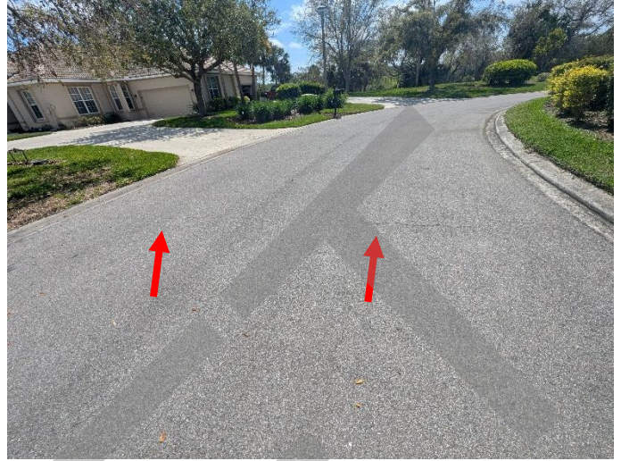
Typical Transverse Cracking – Reserve Ct
