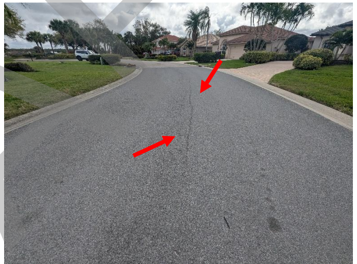
Typical Longitudinal Cracking – Bay Ridge Way
