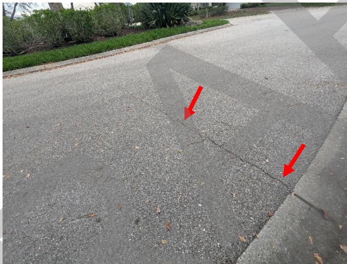
Typical Transverse Cracking – Silkwood Ln
