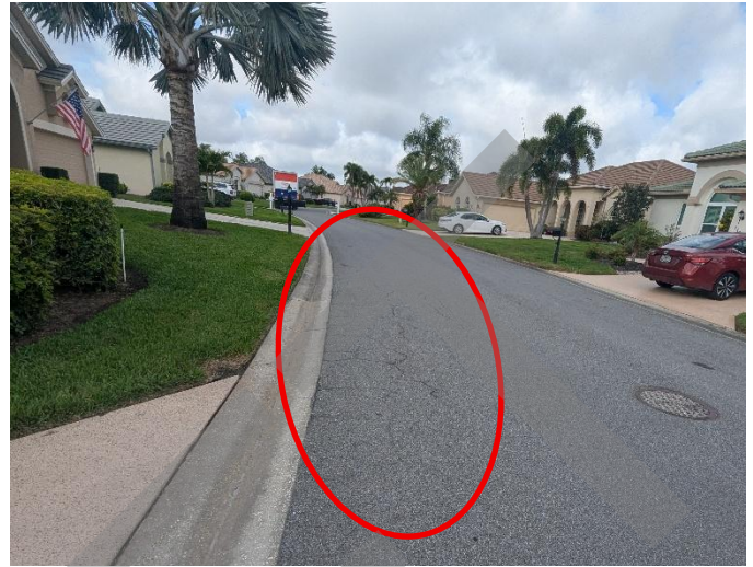
Typical Alligator Cracking – Bay Ridge Way
