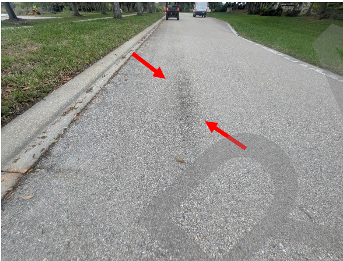
Typical Asphalt Raveling – Club Dr S
