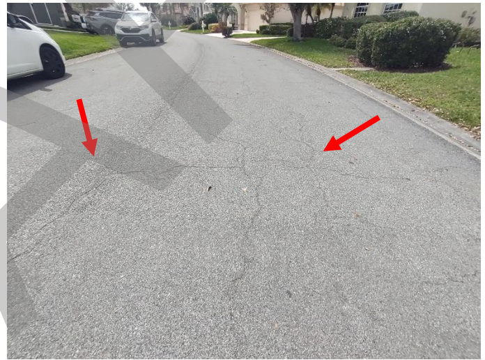
Typical Alligator Cracking – Pennyroyal Rd
