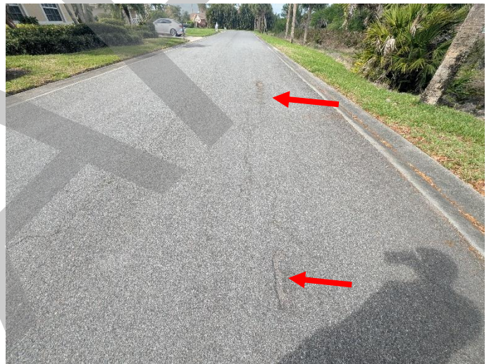
Typical Asphalt Damage – Bay Ridge Way
