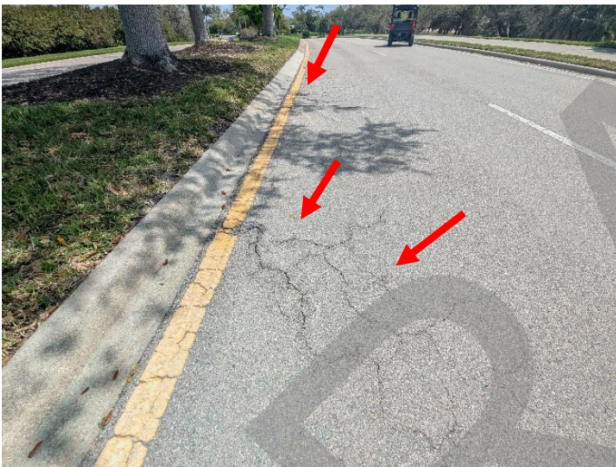
Typical Edge Cracking & Root Damage – Riverwood Dr
