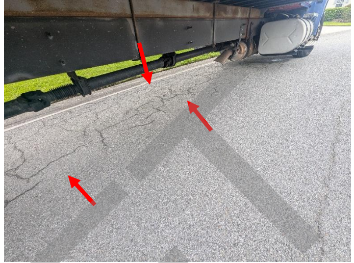
Typical Alligator Cracking – Bay Ridge Way
