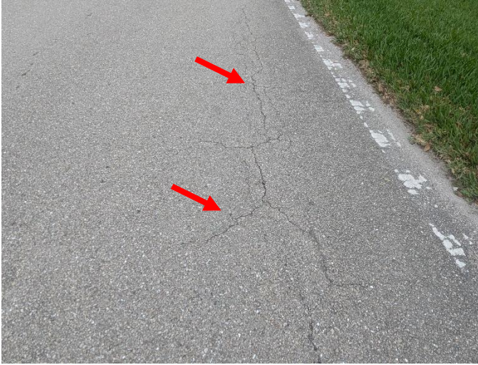
Typical Alligator Cracking – Club Dr S
