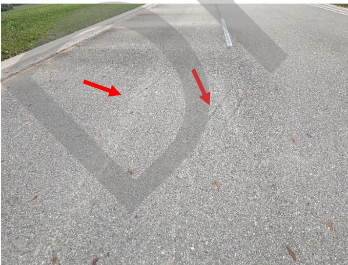
Typical Asphalt Damage – Willow Bend Dr
