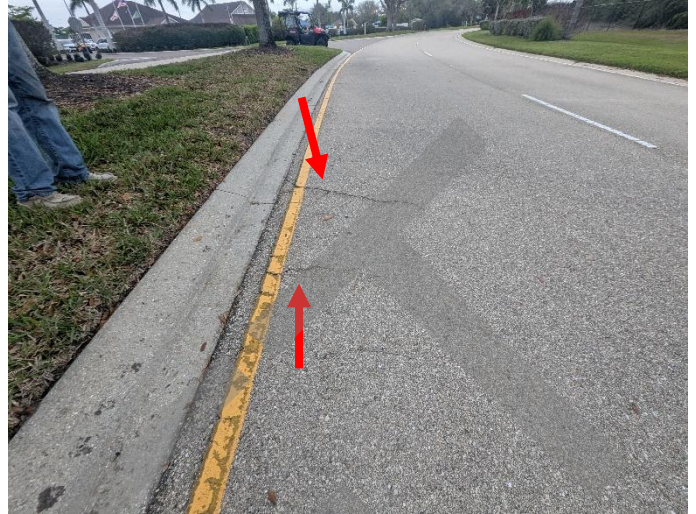
Typical Edge Cracking & Root Damage – Willow Bend Dr
