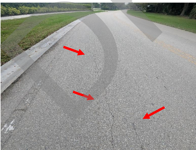
Typical Longitudinal Cracking – Club Dr S
